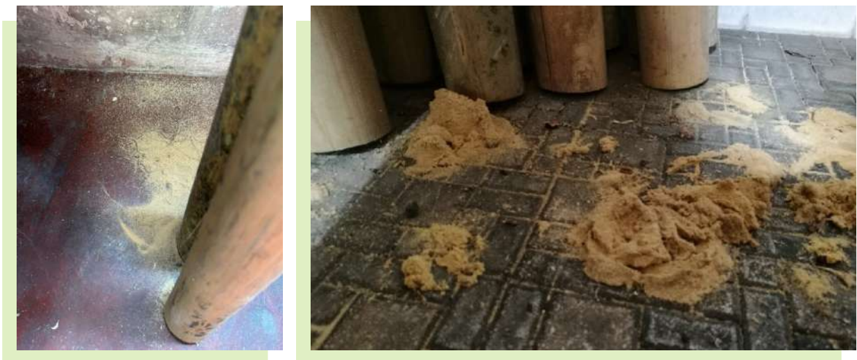
Figure 10. Defective bamboo logs with powdery dust from bamboo holes after insect infestation © Chuen Mun Wai
