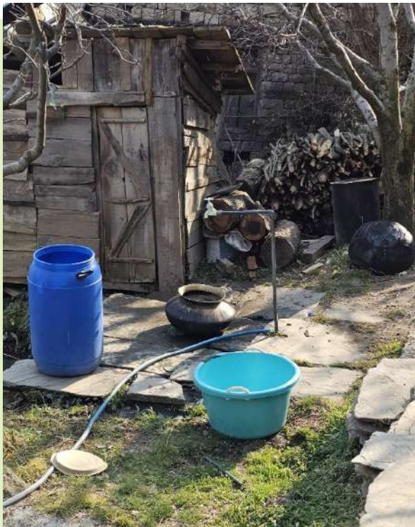
Figure 5. Water pipelines for tap water, installed at Shaleen eco village © Madhusudan Singh
