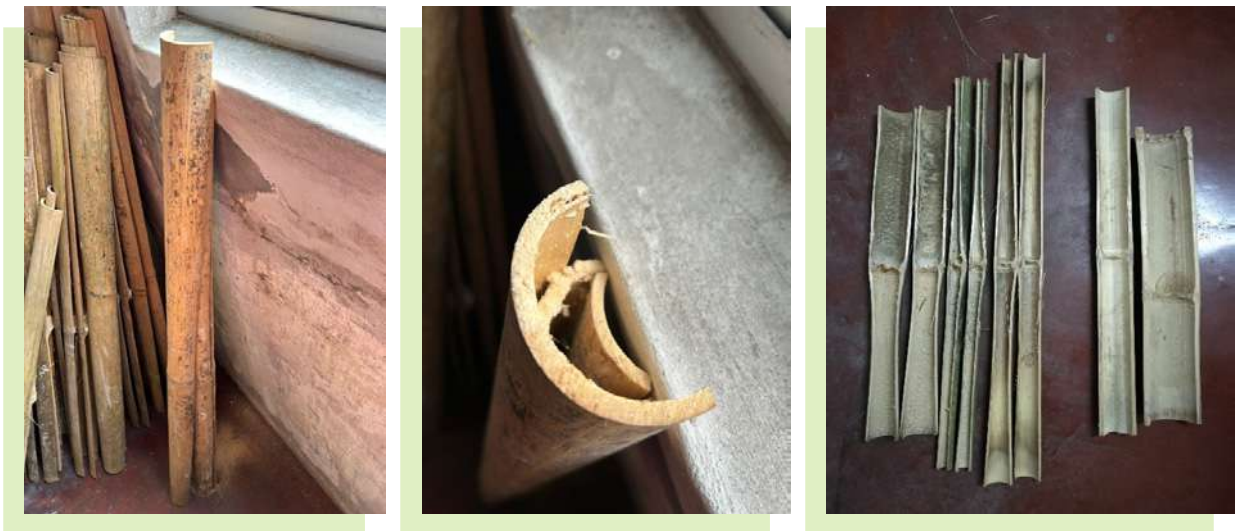
Figure 8. Defective bamboo logs with cracks, ruptures and splits, and irregular shapes. These defects are were probably due to excessively high temperatures or sudden temperature fluctuations, which caused irregular drying during the six-month drying process © Chuen Mun Wai
