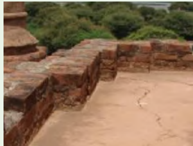
Cracks in the roof of a temple, Bagan, Myanmar, 2016. Photo: Eugénie Crété.
