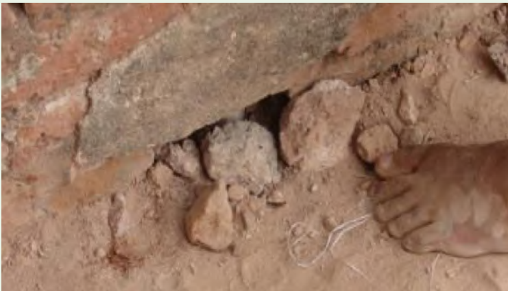
Holes in the roof waterproofing system of a pagoda in Bagan, Myanmar, 2016. Photo: Eugénie Crété.
