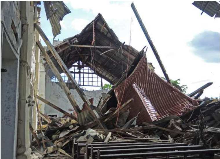
A church damaged by earthquake in Bohol, Philippines, 2013. Photo: Aparna Tandon, ICCROM.
