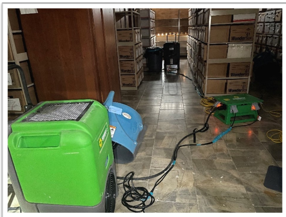
Image 9. Dehumidifiers and ventilation fans. (Photograph: Emilie Gagnet Leumas.)
