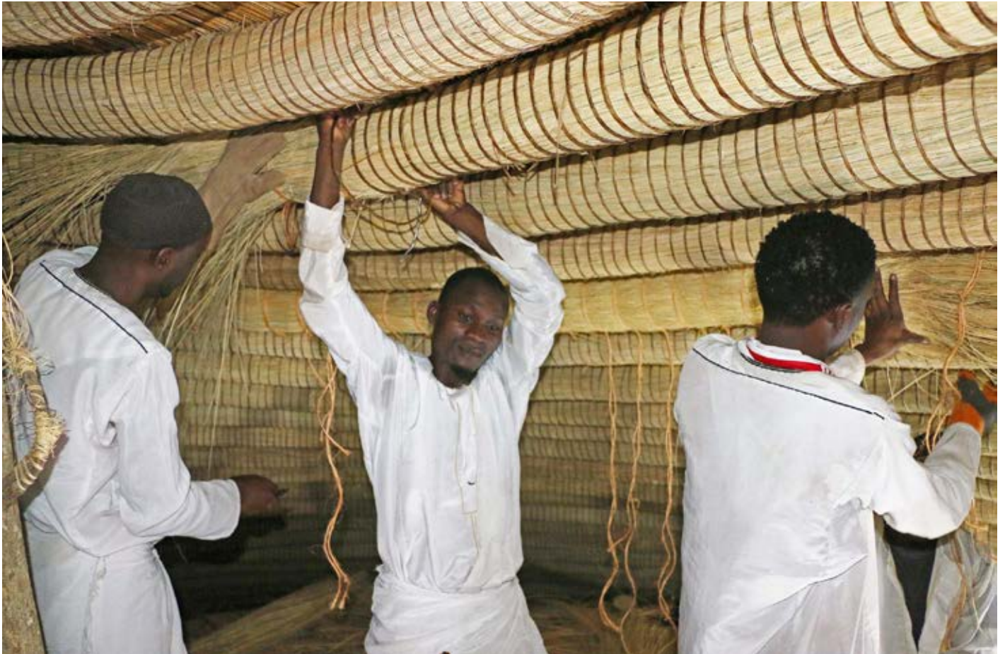
▼ Craftsmen install reed rings to support the thatched roof of one of the buildings on the site.
