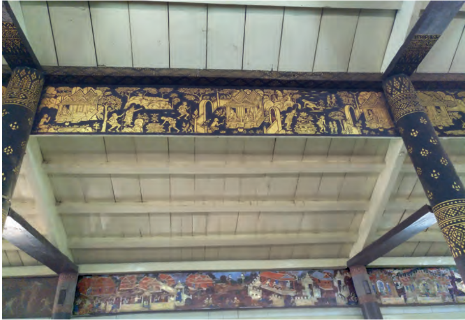
Location of the panels on the beams of the teaching hall at Wat Ban Khong
