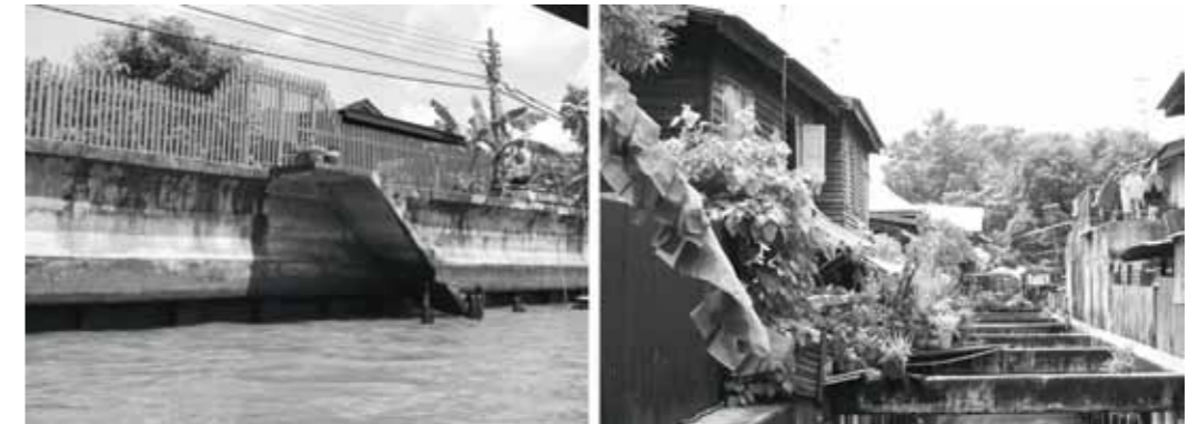
Figure 8. Concrete structures for protection against flooding and erosion cause visual chaos and block transportation
